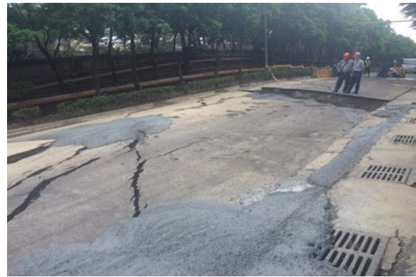
Figure 6. Alligator cracking of the road that occurred due to the land subsidence hazard.
