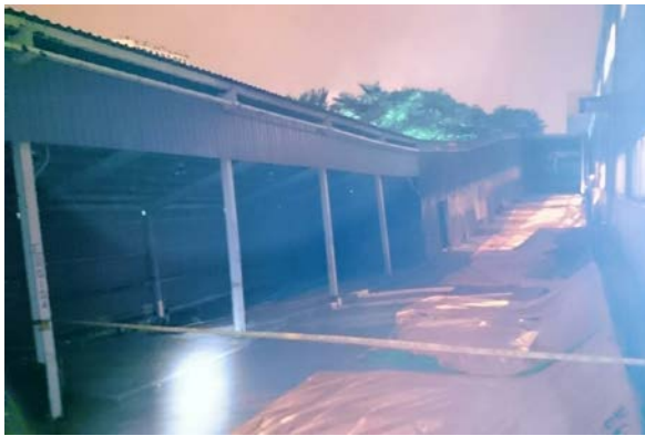
Figure 5. The CPC warehouse subsided due to the land subsidence hazard.
