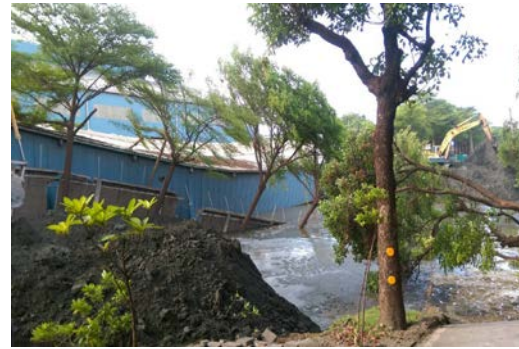
Figure 3. Warehouse subsidence due to subsurface settlement.
