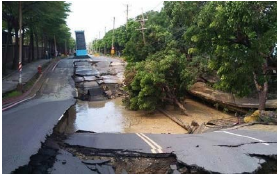
Figure 2. Road subsidence due to subsurface settlement.
